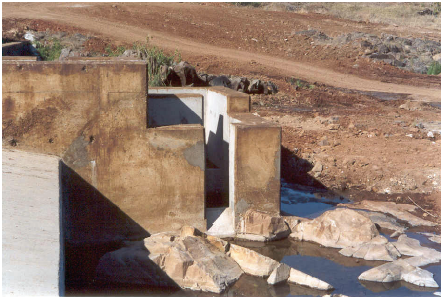
Plate 3.4: View of most downstream slot of the “Pool and Slot” Ten Bosch fishway on the Crocodile River in the KNP, during low stream-flow conditions (no flow through fishway).
