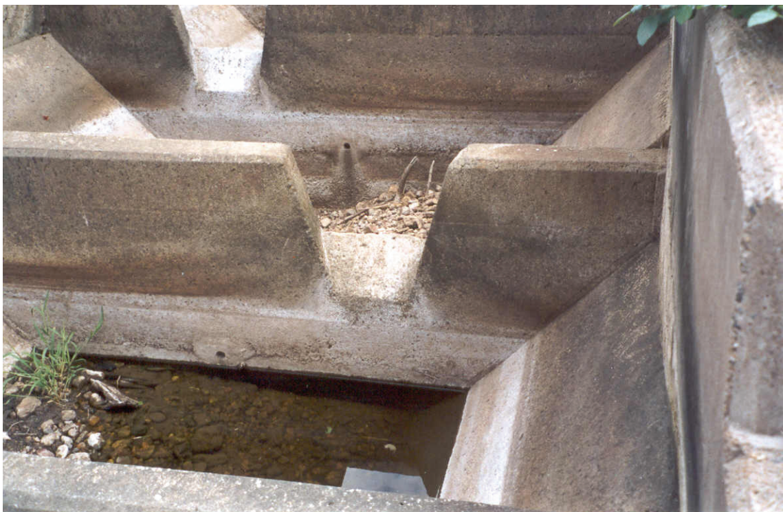
Plate 3.2: Close-up view of weir notch in the Kanniedood fishway, KNP during low-flow conditions.
