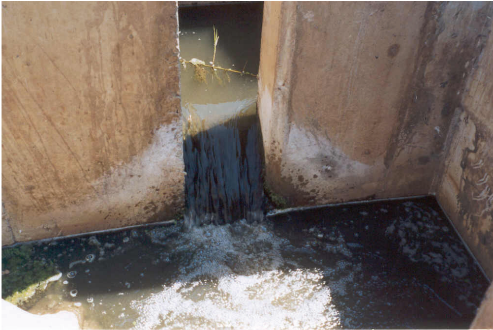
Plate 3.5: Close-up of “Pool and Slot” baffle at Riverside Weir fishway in the KNP under low flow conditions.
