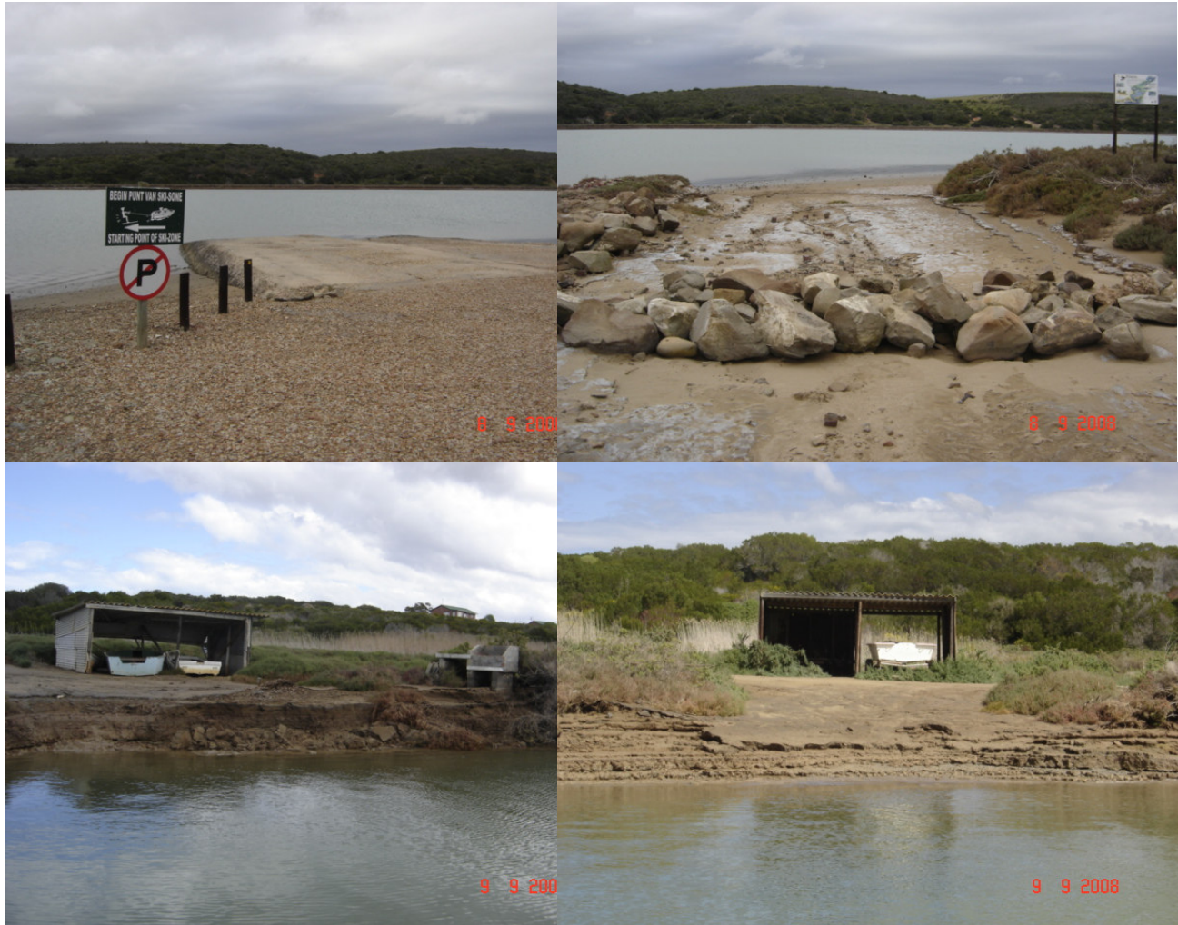
Plate 7.2 The existing slipway and car park (top left); the old slipway (top right); the two boathouses and slipway located on the west bank in the middle reaches with bank erosion (bottom left and right).
