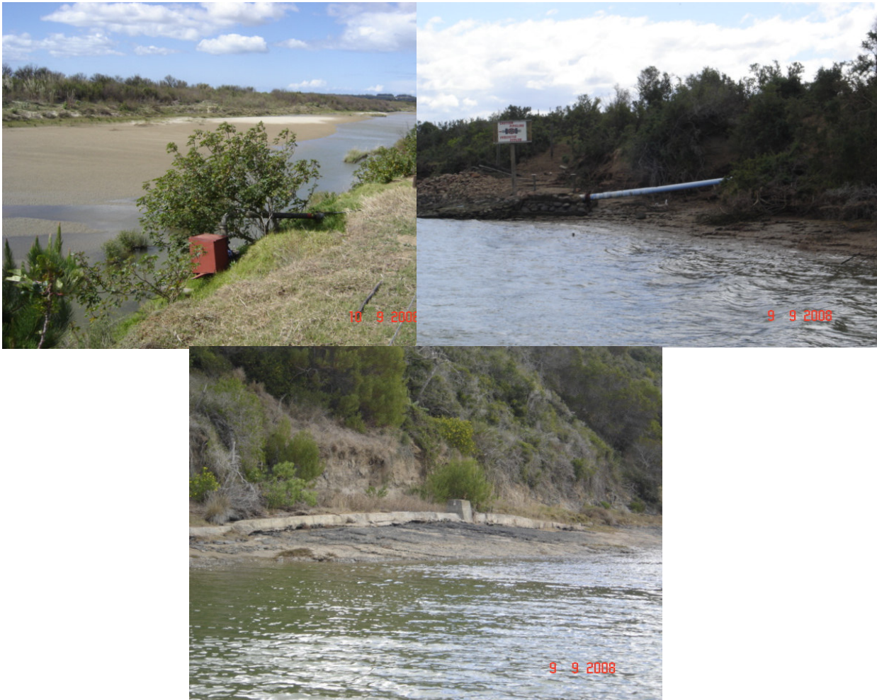
Plate 7.5 Two pumps located in the lower region of the river (top left); water pipelines that span the width of the estuary in the middle reaches (top right); and a protected pipeline running alongside the middle reaches of the estuary (bottom).
