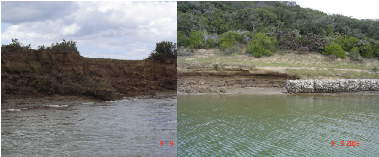
Plate 7.4 Erosion of a section of the eastern bank in the middle reaches (left) and stabilization attempts using gabions with the resultant downstream erosion (right).
