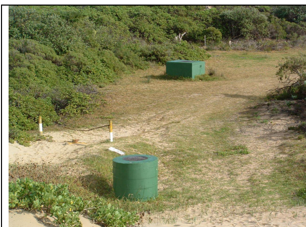
Figure 5. Wells for the abstraction of seawater near the mouth of the Bushmans Estuary.
