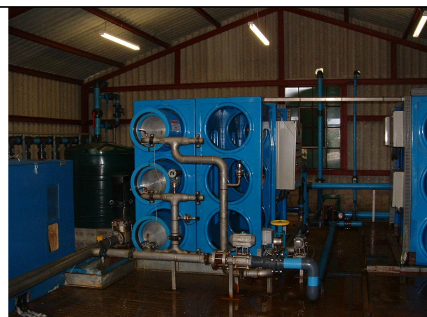
Figure 6. RO3 at the ACWB.
