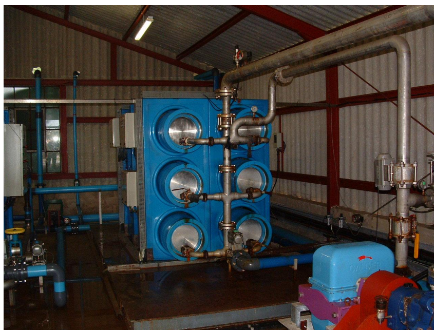
Figure 8. A rack with 6 pressure vessels. The pump is in the foreground right.
