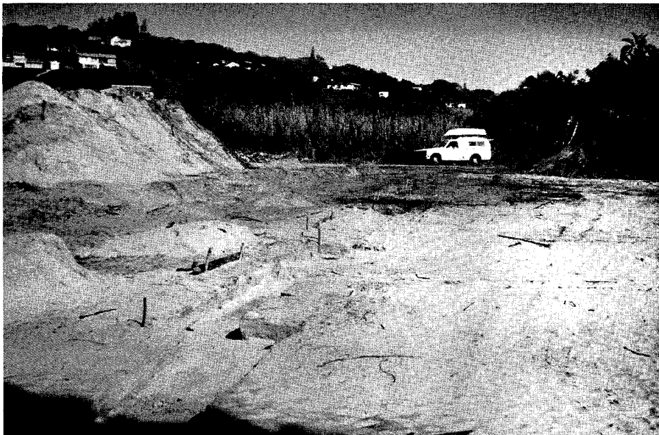
Plate 15: The foundations for a duplex development being excavated in wetlands surrounding the Mbizana lagoon (Ramsgate).
