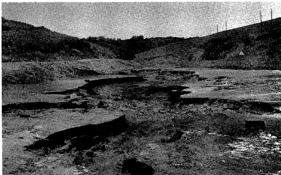
Plate 17b: The remains of the wetlands depicted in Plate 17a after commencing the construction of route MR96 and canalization of the Sweetwaters River.
