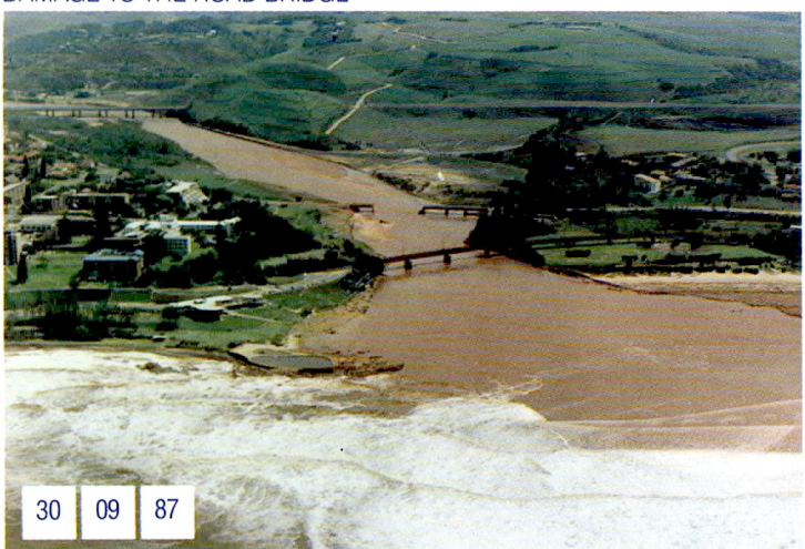
DAMAGE TO THE ROAD BRIDGE
