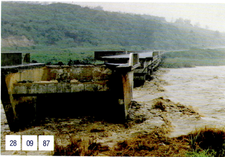
DAMAGE TO THE ROAD BRIDGE NEAR THE MOUTH OF THE MDLOTI, DURING THE FLOOD
