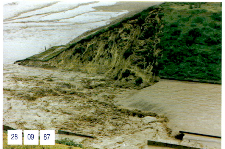
ERODED CANAL OUTFALL
