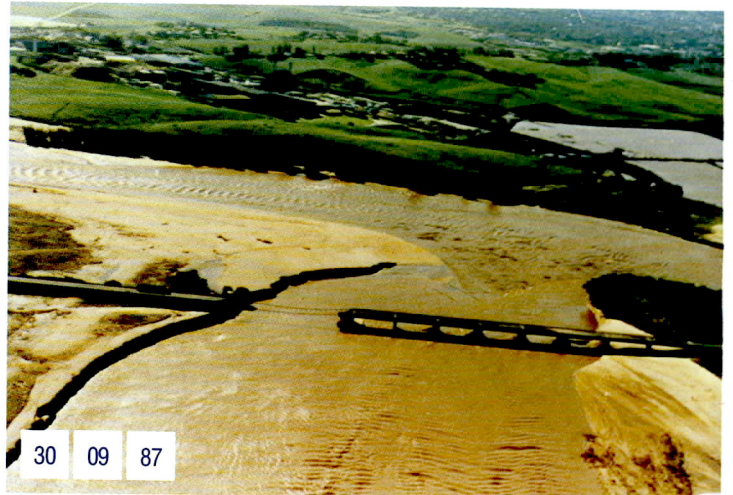
DAMAGE TO THE ROAD BRIDGE 36 km FROM MOUTH
